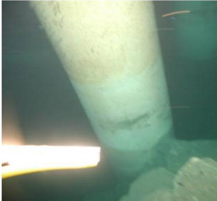
Figure 12 Washed out formation around the well
